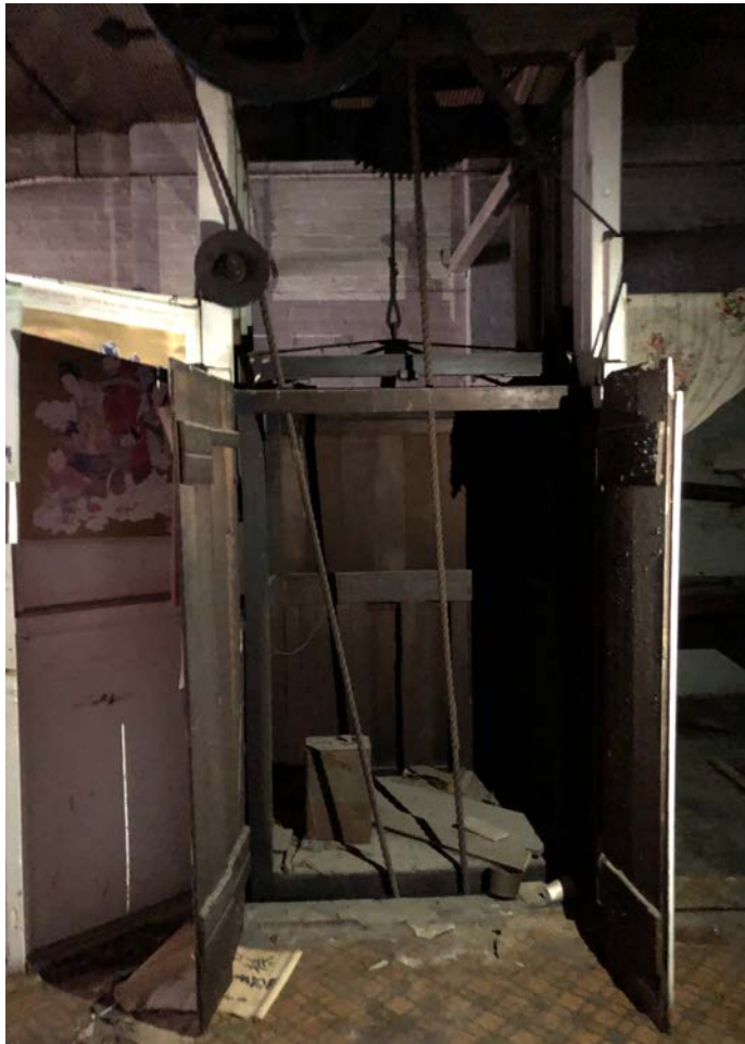
Figure 3: Hand-operated goods lift and assorted ephemera, first floor, 84 Dixon Street.
