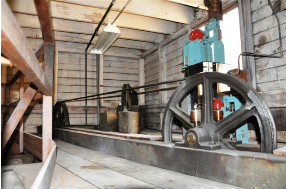
Figure 5: Hydraulic lift cable room (Source: 'Former Shelley warehouse including interiors, NSW Heritage Inventory)
