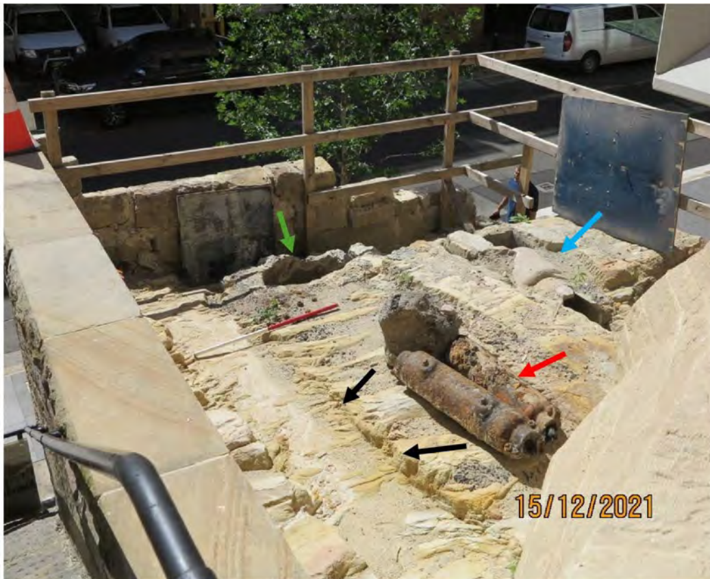
Figure 72 Features identified within the recently excavated garden bed situated behind the sandstone retaining wall along Harrington Street, including stormwater drain (blue arrow), gas pipes (red arrow), and concrete pier base (green arrow). Note the channel through the bedrock where the gas pipe ran (black arrows). View to southeast. Source: Casey & Lowe 2021.
