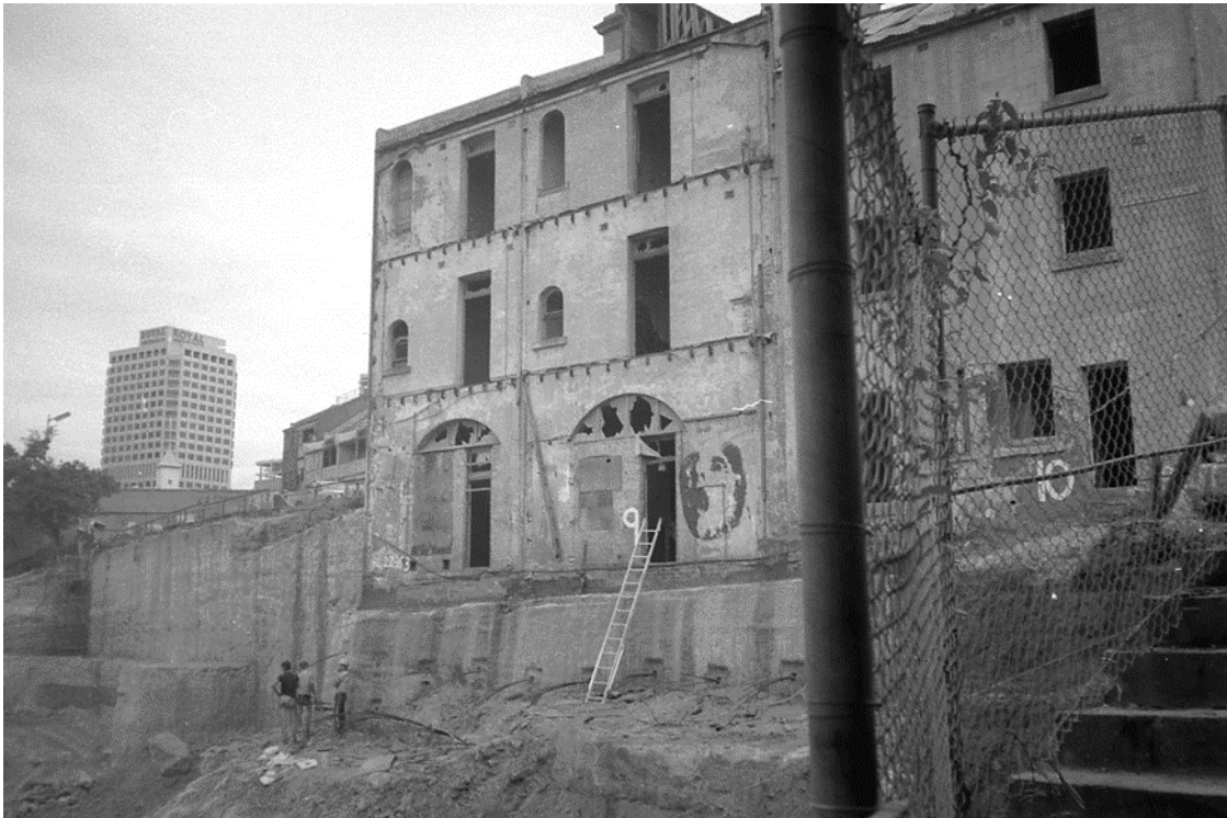
Figure 34 Photo of the rear of Baker's Terrace c. 1988, showing the extensive demolition and excavation which was undertaken at the rear of the buildings and the excavation in this area of the Cumberland Place.
