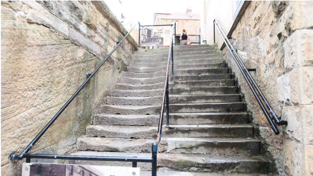
Figure 66 Staircase A. The concrete capping has been removed on the southside but remains on the north.
