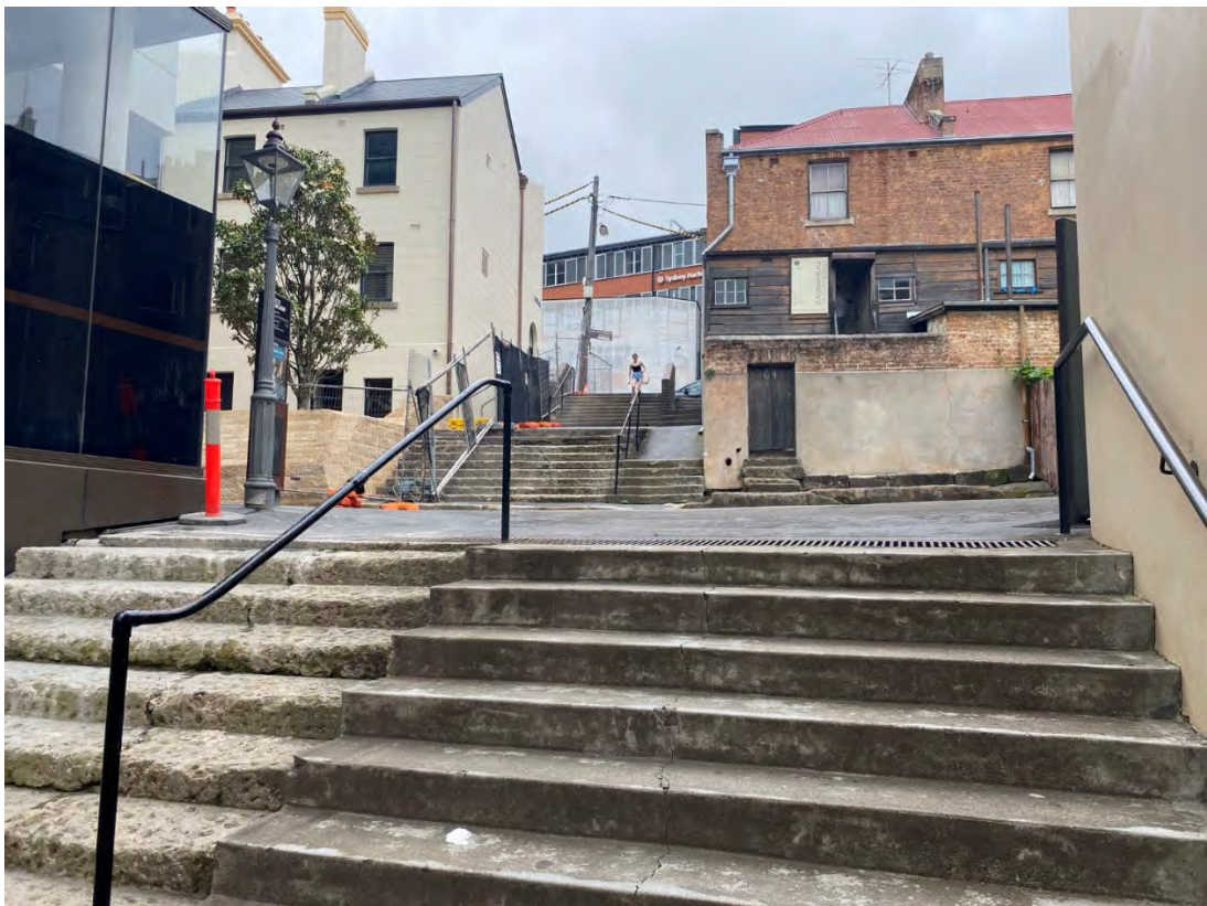
Figure 67 Staircase B. The concrete capping has been removed on the southside but remains on the north.
